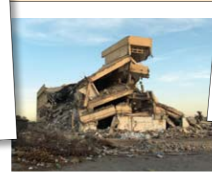
Damaged building in Tripoli
